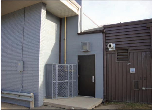
Unintended access to the roof at the rear of a property due to the placement of screens and roof overhangs.
